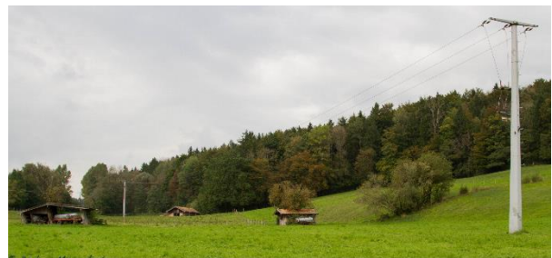
Fig. 8: At this power line in Piding, Germany, four Northern Bald Ibises were electrocuted at the same time. In contrast to the regulations, the power line is unsecured; Photo by B Aichner.
